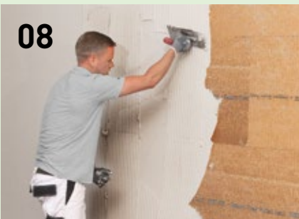
Fill the entire surface of the insulation panels attached to the wall using a toothed trowel and PP Fill.
