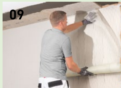
Using the smoother, integrate reinforcement fabric in the reinforcing mortar using overlapping, crease-free vertical strokes.
