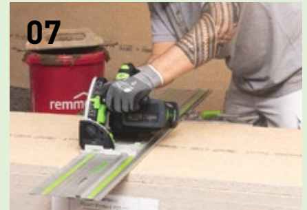
Cut the wall connection panels to size using the Festool TSC 55 and guide rails. Where necessary, sand down any protruding joints with the ETS EC 150/5.
