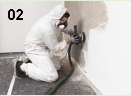
Remove defective areas of plaster and old coatings using the renovation miller or the surface-restoration grinder.
