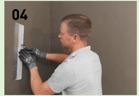
Level off (up to 8 mm) the substructure using adhesive mortar PP Fix and a wide filling trowel.
