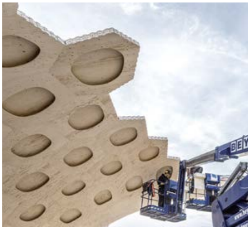
→ The hollow tile segments were partially pre-assembled and put together on site without substructures or a support frame.
